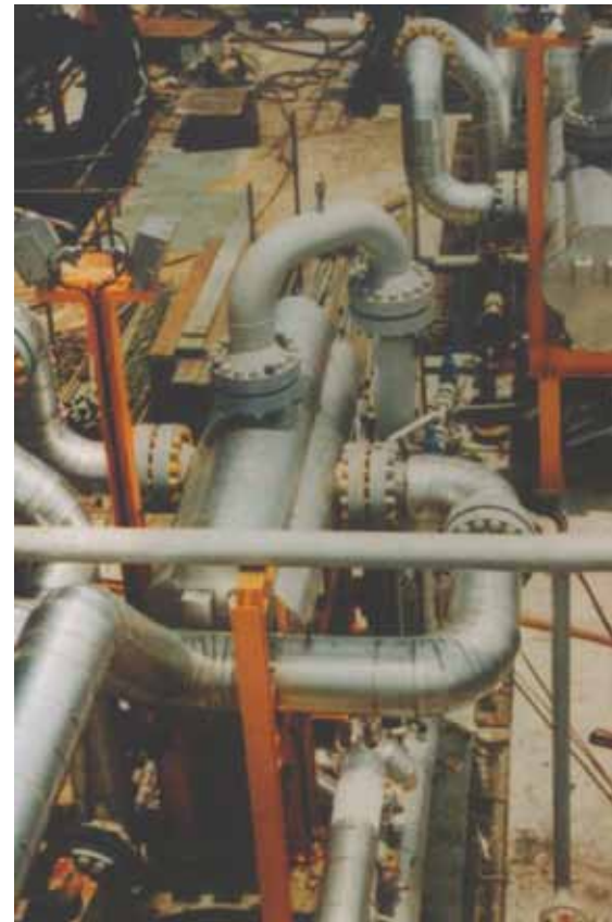
PCHE installation on a South China Seas platform
